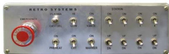
Operator control panel for (4) stations
